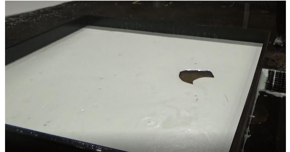
Non-aspirated sprinkler test failure after water deluge
