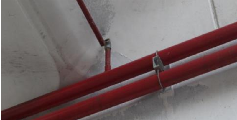
Excessive relative movements/rotations between pipes
