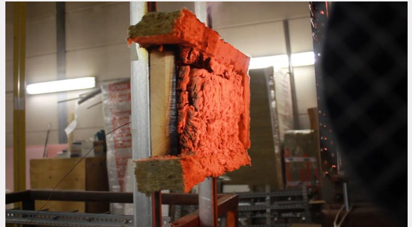
Delamination: lamella falls off (ME glue)
