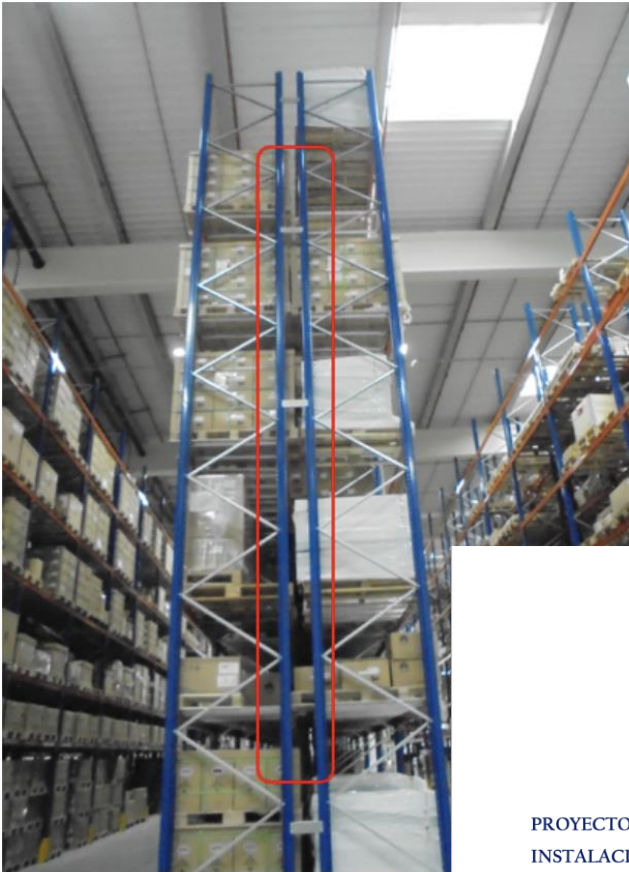
Absence of longitudinal aisle
