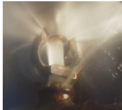
Spray obstruction by sealing
