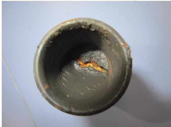
ESFR K25 (2002) dirt at sealing
